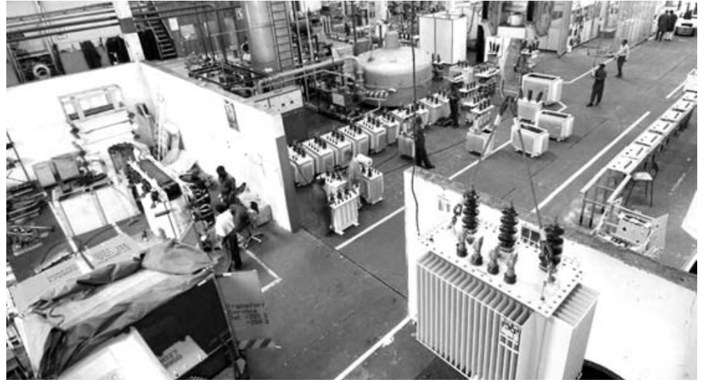
TransCentury generates private equity returns through investing in fast-growing sectors in Africa with companies such as Tanelec Tanzania, the largest manufacturer of electrical distribution transformers in East and Central Africa. Tanelec was recently awarded the President's Manufacturer of the Year Award in Electrical Machinery, Equipment and Electronics
